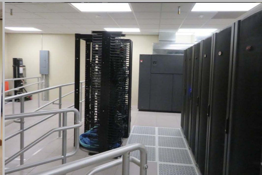
DEDICATED IT SERVER ROOM
