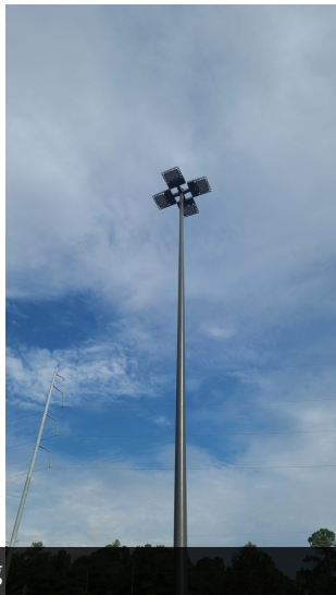
New LED parking lot lighting
