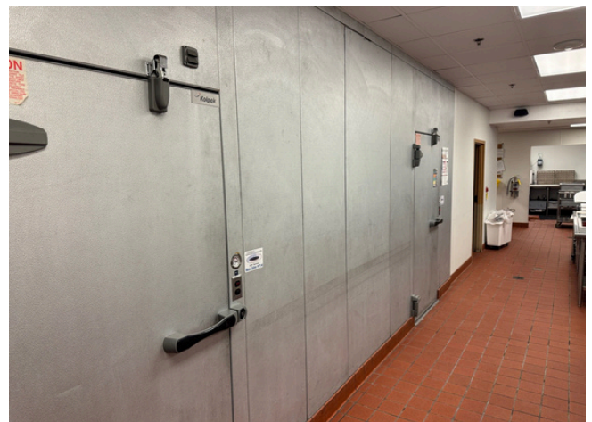
Large Walk-in Freezer and Refrigerator
