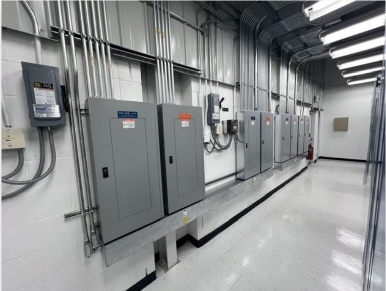
Electrical distribution panels
