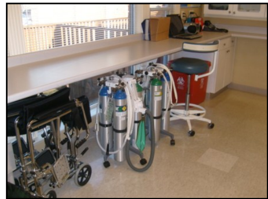
16 : Oxygen and nitrous oxide gas cylinders
