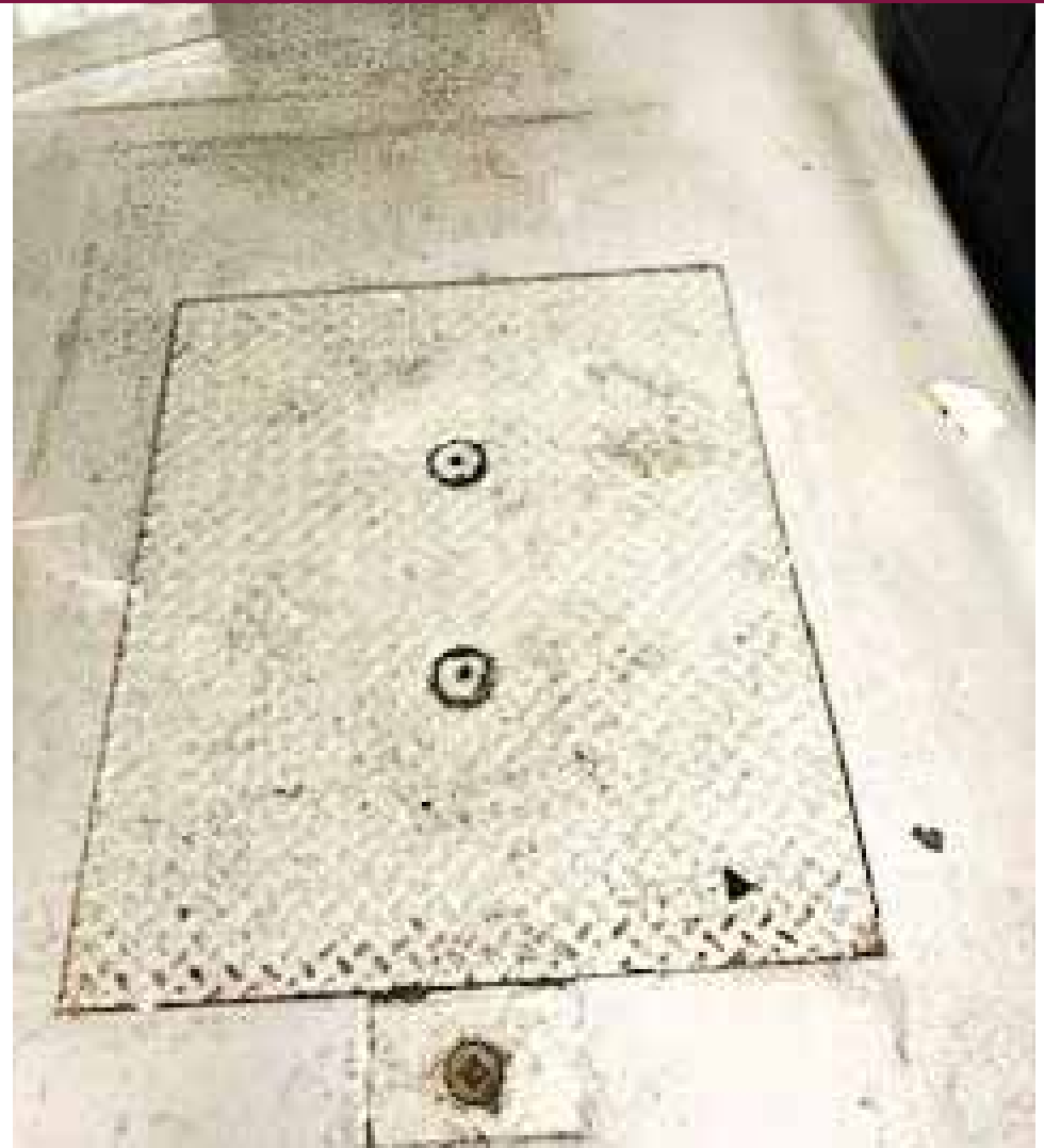
In-Ground Grease Interceptor
