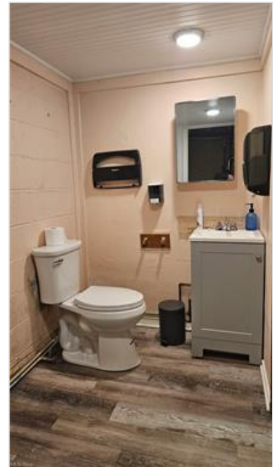
Bathroom with wood finished floors, vanity, concrete block wall, and wooden ceiling
