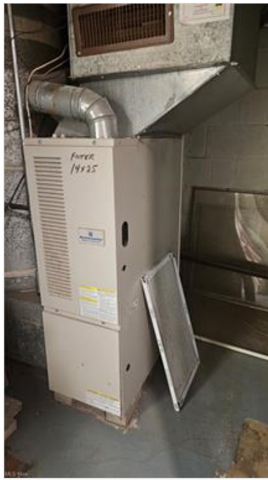
View of utilities
