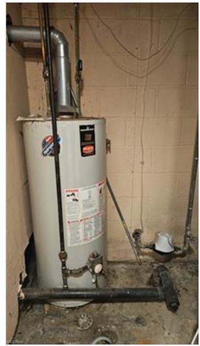
Utilities featuring water heater
