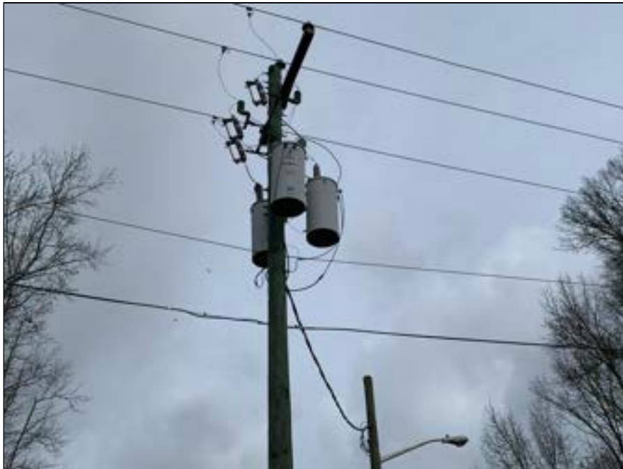
12 - View of pole-mounted electrical transformers located on the north side of the stream separating the Property from the residential properties located to the north.
