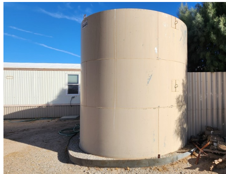
According to the tank tag: used for Potable Water only; 10,000 gallon capacity; manufactured in 9-99 by Tiger Tanks, Inc.
