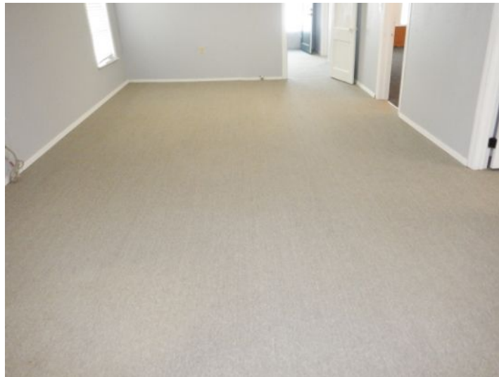
There are indications of floor slope.
