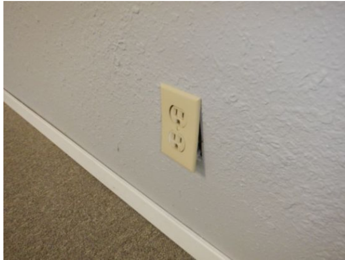
There is a loose electrical outlet in the family room.
