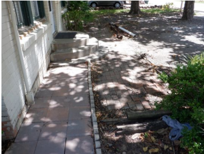
There is concrete settlement at the walkway. This is considered a trip hazard.
