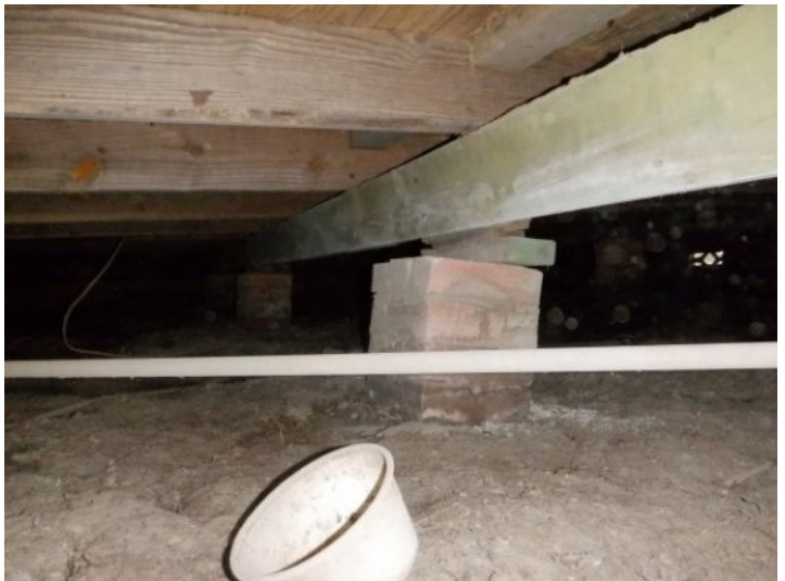
The foundation support blocks have shifted. The blocks do not provide maximum support under these conditions.
