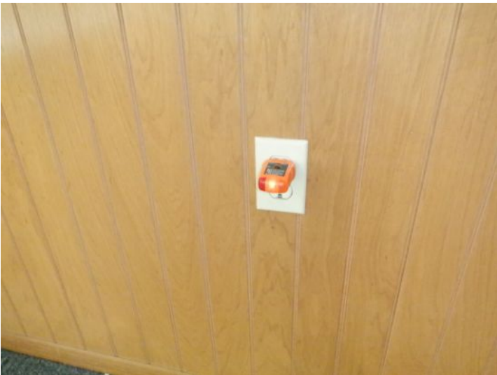
There are electrical outlets that measure open ground.
