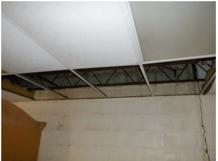
There are missing and damaged ceiling tiles.
