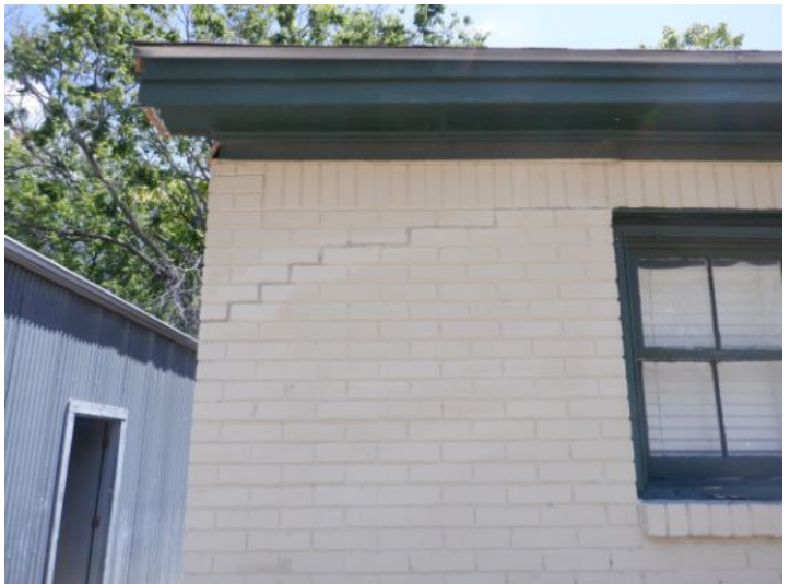
There are exterior cracks along all sides.
