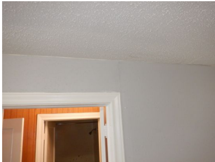
There are interior drywall cracks at most rooms.
