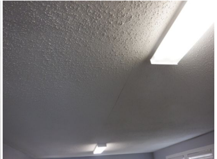
Cracks in the interior drywall ceilings were noted at the family room.
