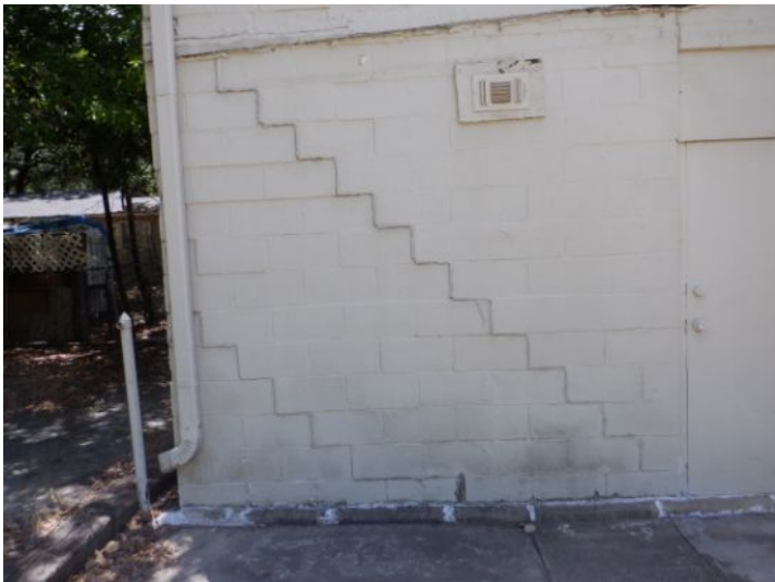
There are exterior cracks along all sides.
