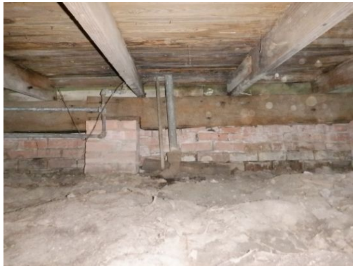
The foundation wall is failing near the rear of the structure.
