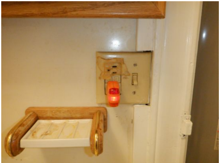
The GFCI (Ground Fault Circuit Interrupter) electrical outlet did not reset in the bathroom.
