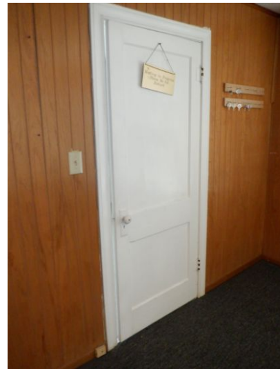
There are doors that will not latch at the bedroom and bathroom. Recommend adjustments.
