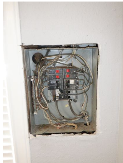
Main service panel with cover removed photograph
