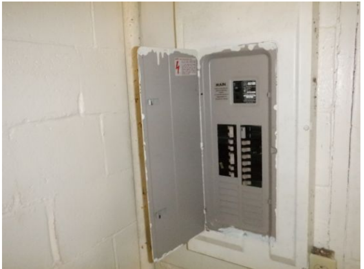
There was no power to the structure at the time of inspection.
