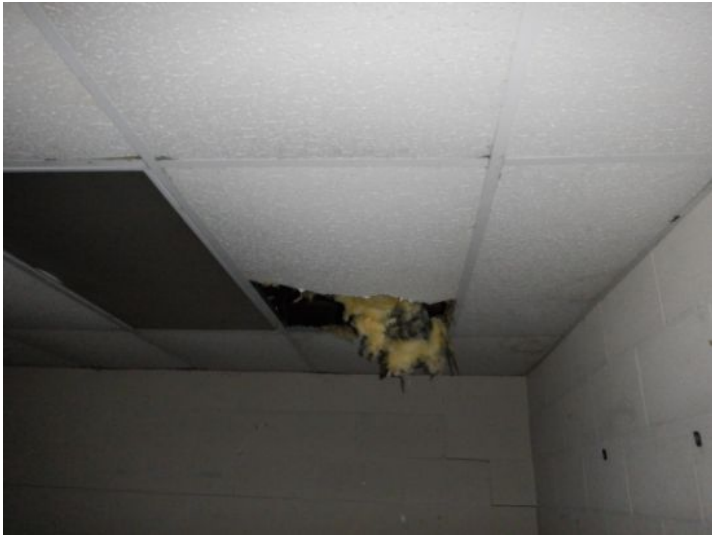
There are missing and damaged ceiling tiles.
