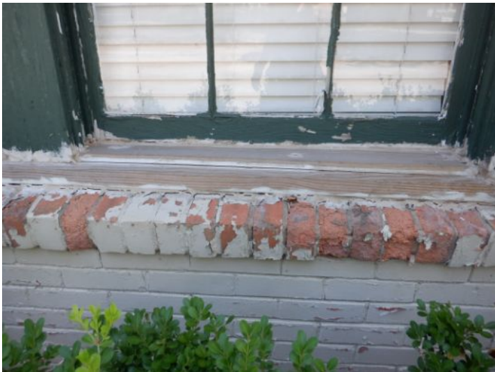
The siding and trim was unsealed or unpainted along the windows. Unpainted siding and trim has no protection from the environment.
