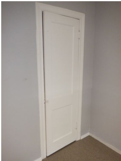
There are doors that will not latch at the bedroom and bathroom. Recommend adjustments.
