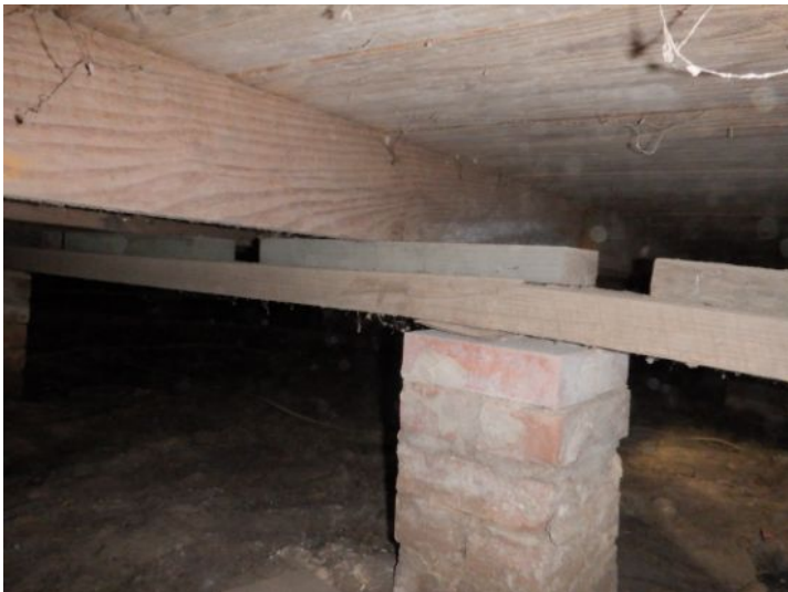
The foundation beam is laid horizontal. Beams should be laid vertically to provide maximum support.
