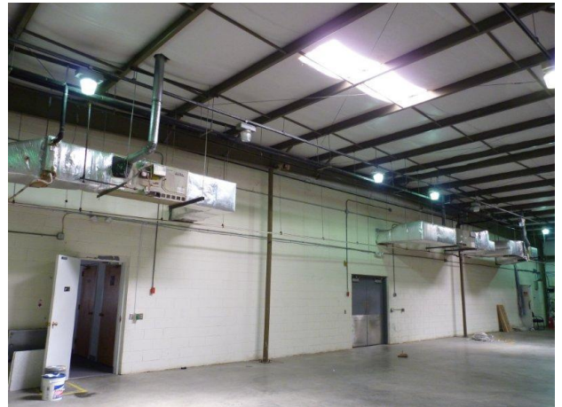
SKYLIGHTS, GAS FIRED HEAT PUMPS FOR OFFICE AREA
