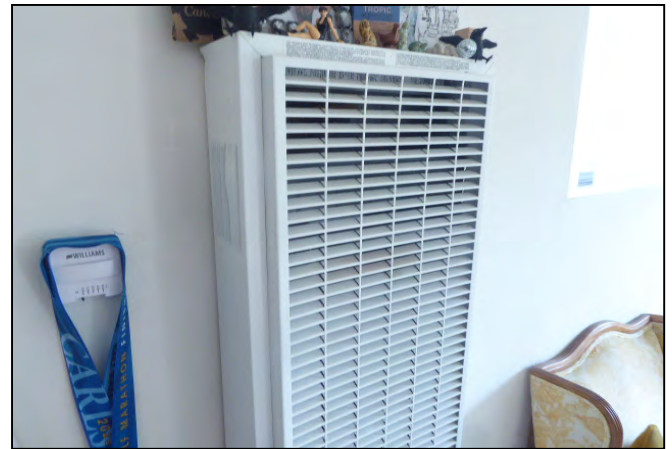
Unit 432 – Wall Heater
