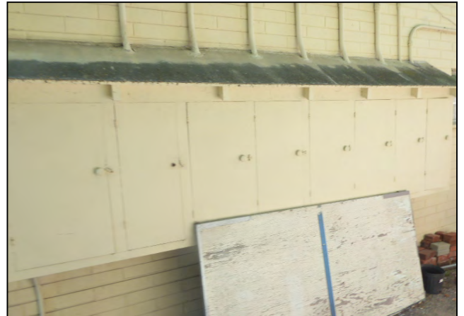
Electrical Meter Cabinet
