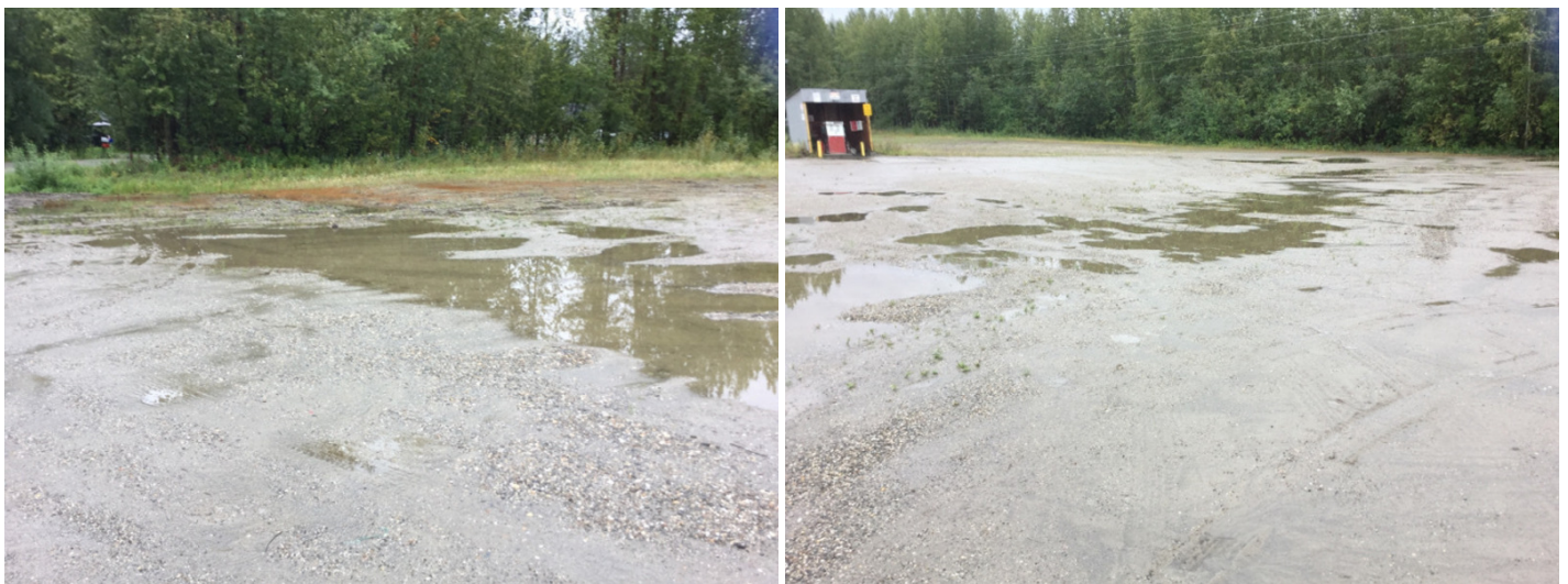
Grading, Drainage, or Flooding Issue Photos
