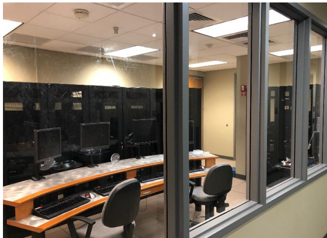
Secured Data Center
