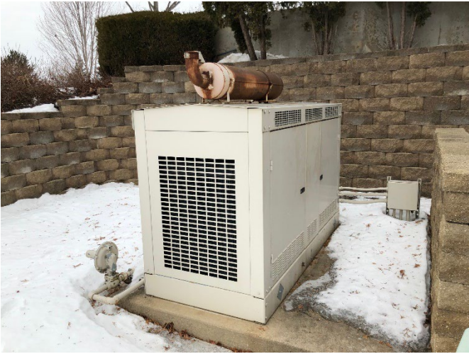
81 Kw Spectrum Brand Generator
