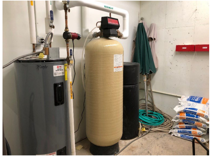
Water Softening System
