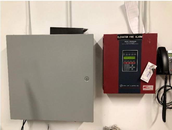
Fire System Panel
