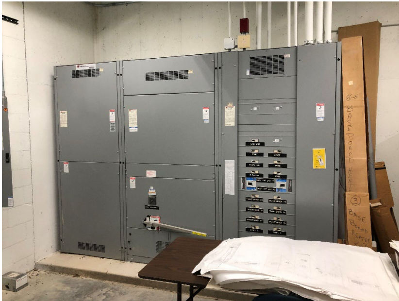
Main Electrical Switch Panels
