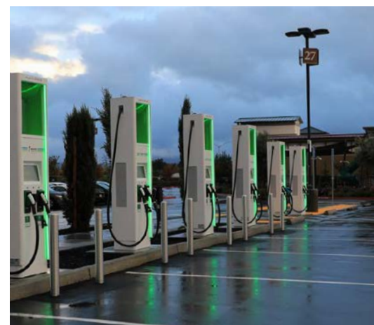
Electric Car Charging Stations
