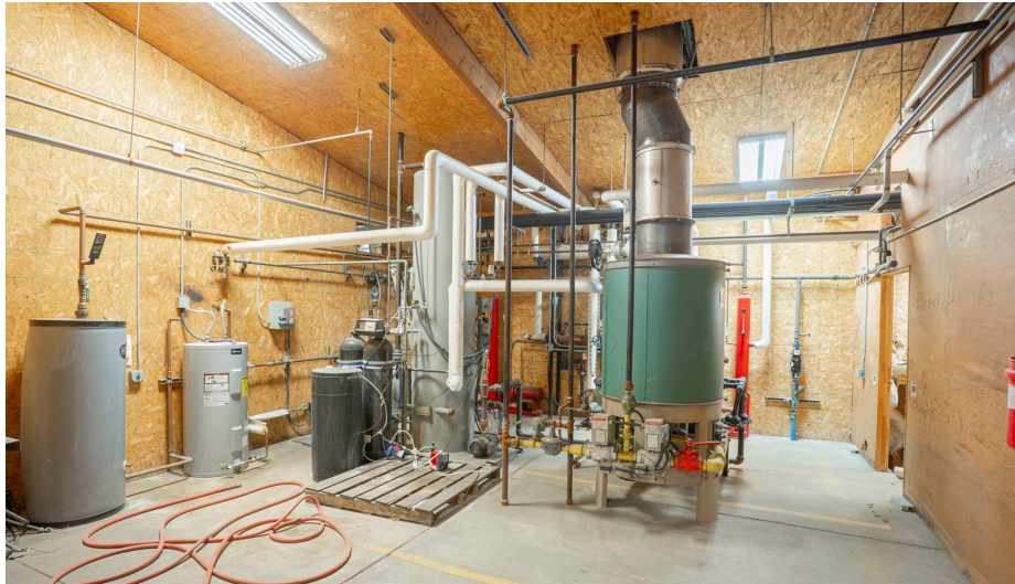
BOILER & EQUIPMENT ROOM
