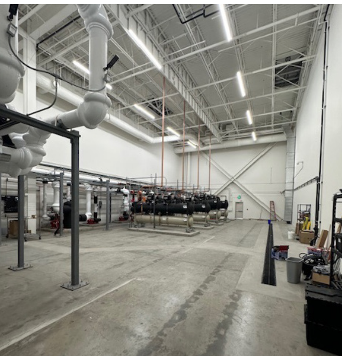
MECHANICAL ROOM (PUMPS, HVAC, CLEAN ROOM SUPPORT ROOM)
