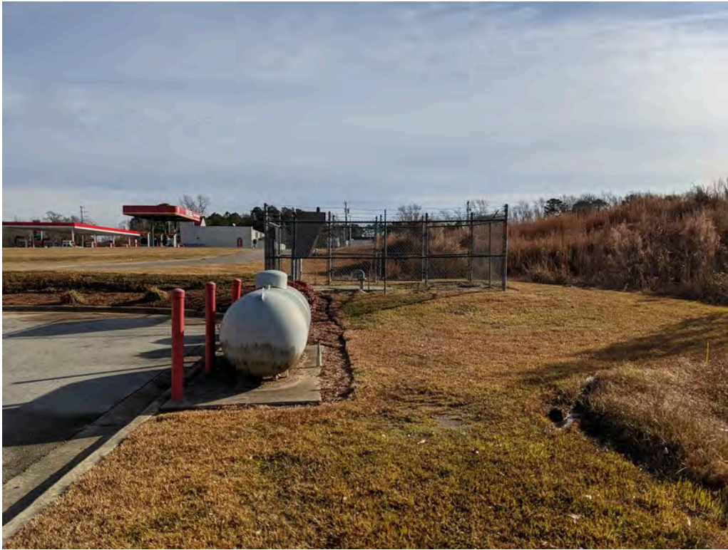
Propane AST and sewer lift station located on the Subject Property, south of the carwash property
