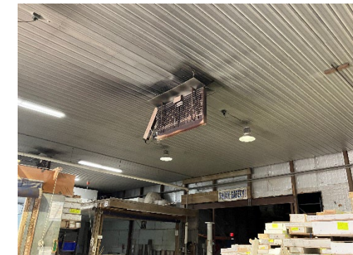
Radiant heaters in production area
