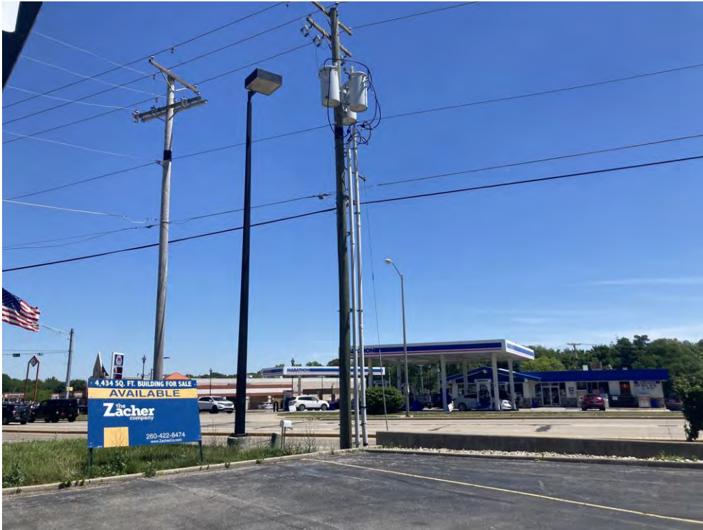
Photo 13: Transformers at the southeast corner of the property
