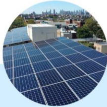
Roof Solar Panels
