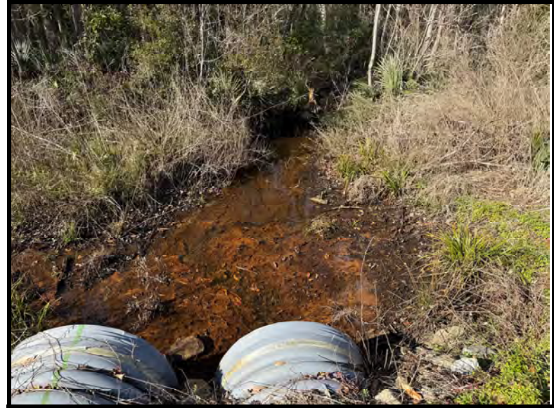
6 Tributary facing northwest from the existing bike trail in the southeastern portion of the property.
