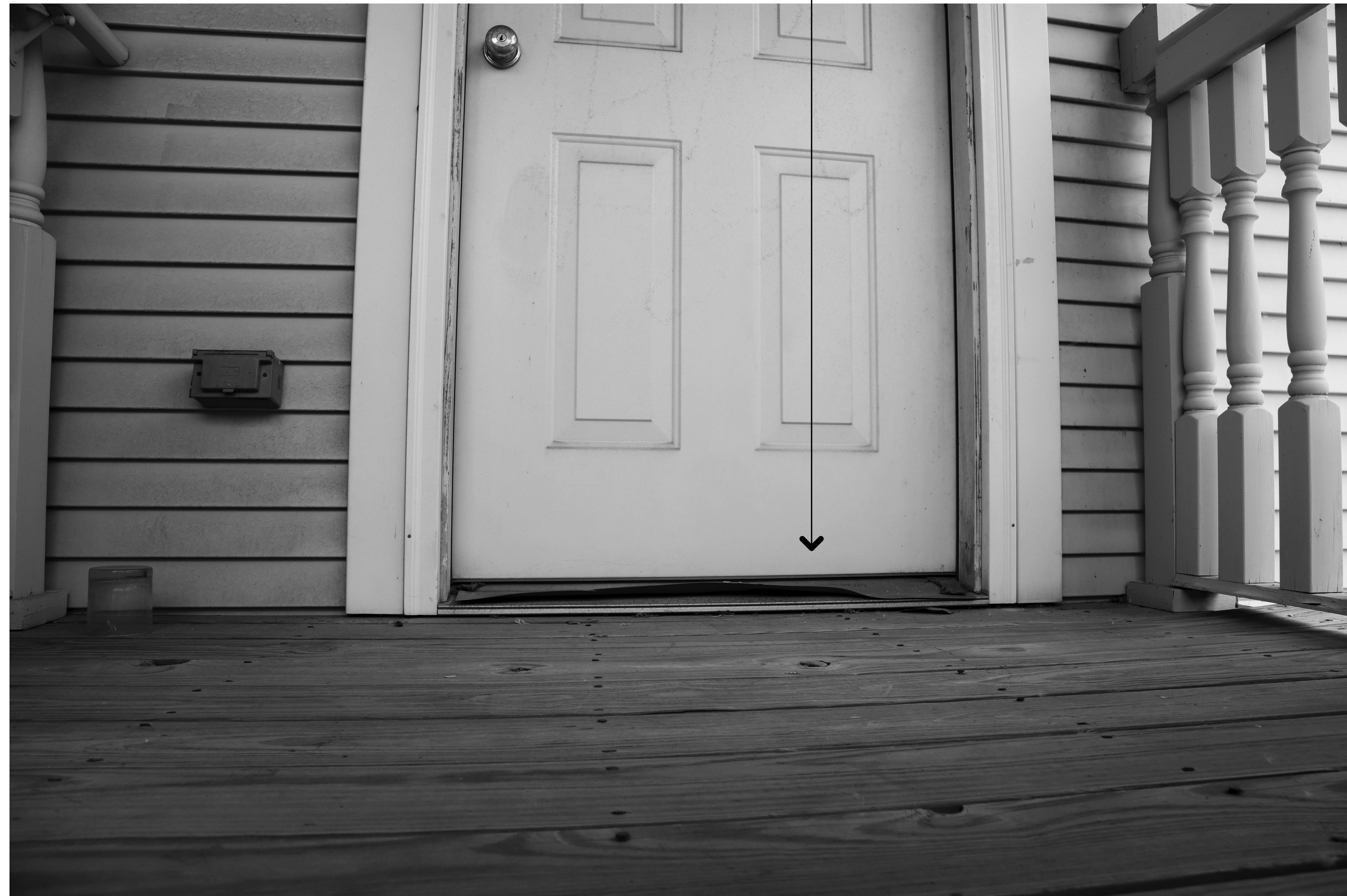
Existing Second Floor Egress Door Thresholds
