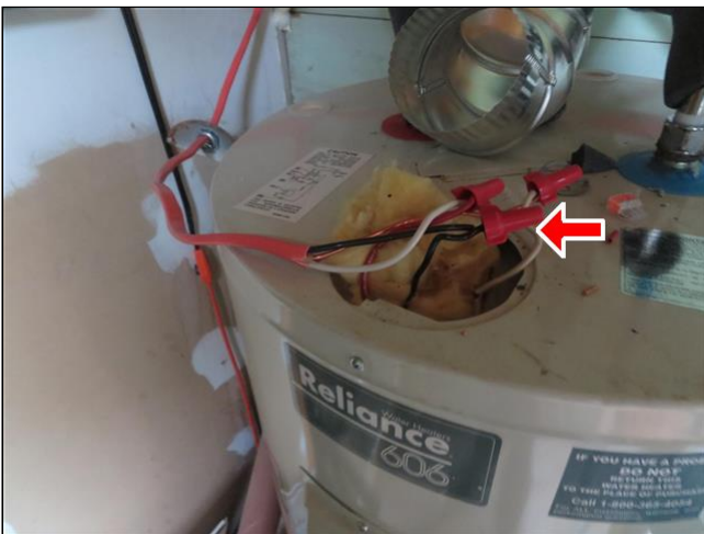
7.3 Item 3(Picture) Utility room
