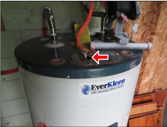
7.3 Item 2(Picture) Utility room
