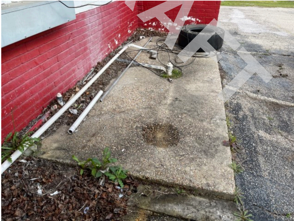
14. Evidence of grease trap
