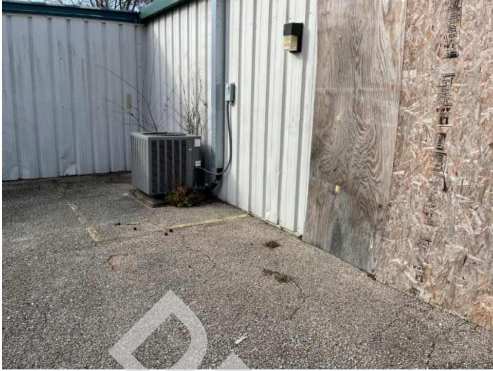
13. HVAC condensing unit at office building
