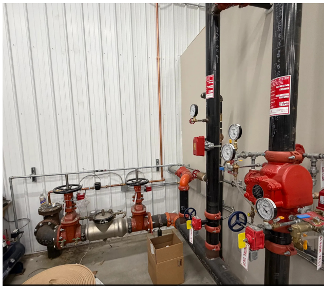
Full sprinkled, dry system in attic, wet below
