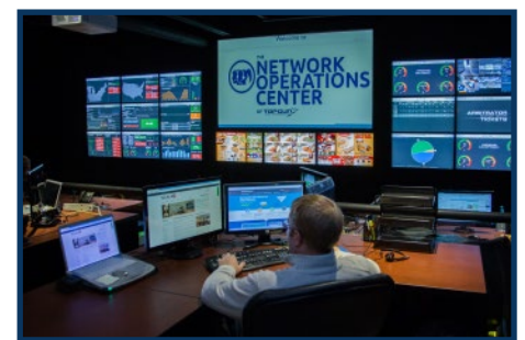
Network Operations Center
