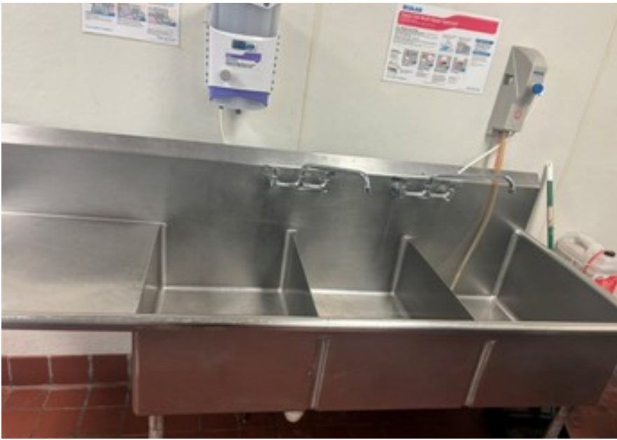
Three Compartment Sink Station
