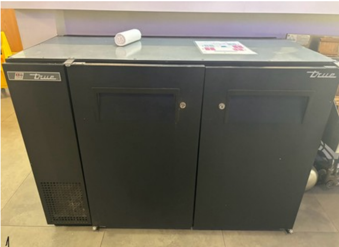
Under-counter Refrigerator #1 ( Deactivated and not working, needs to be repaired)
