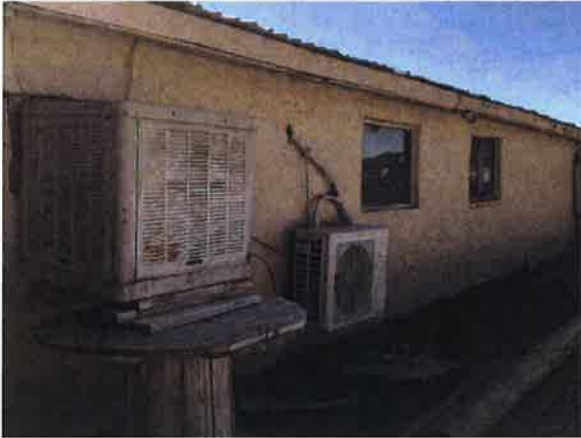
Evaporative cooler and heater
