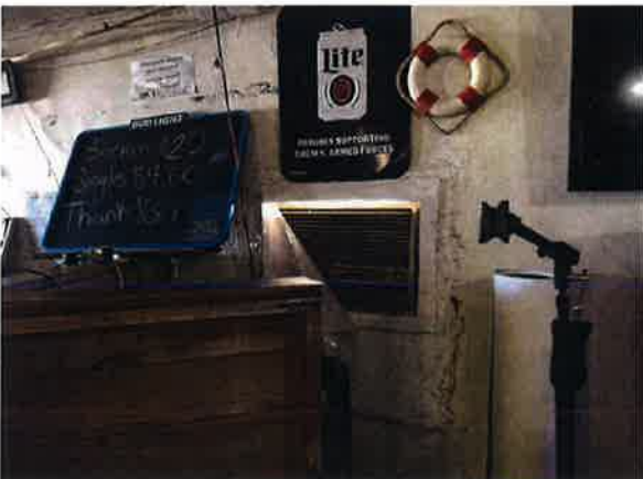
Refrigerated Air Window Unit Used to enhance the Central Evaporative Cooling
