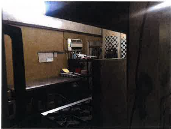
Kitchen Gas Stove top
