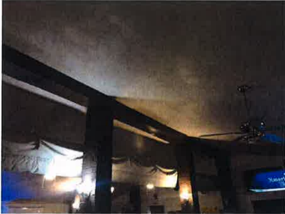
Ceiling Air Vents and Ducting and columns
