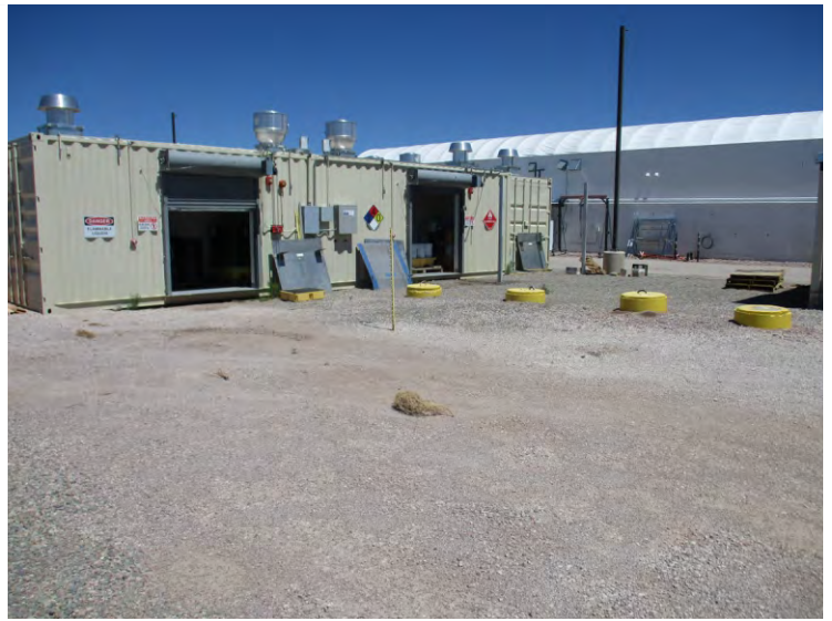
Photo 34 - View of the waste storage buildings and septic tank covers west of Greenhouse 1, looking northeast.
