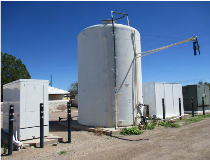
Photo 9 - View of the water tank, emergency generator and transformers south of the White House, looking northeast.
