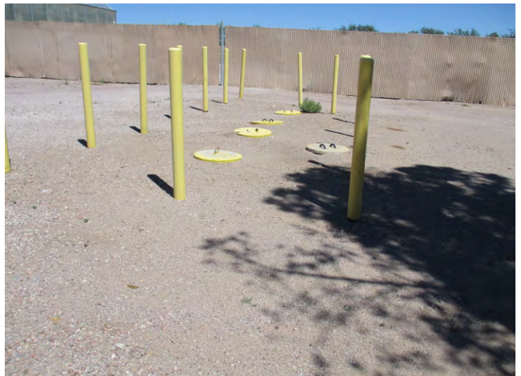
Photo 14 - View of septic tank covers north of the White House, looking north.
