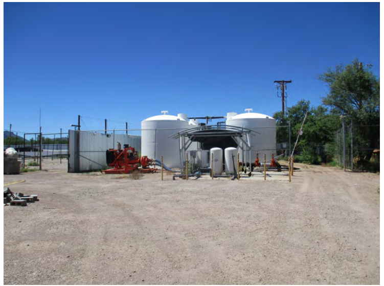
Photo 28 - View of the water well complex on the west portion of the subject property, looking west.
