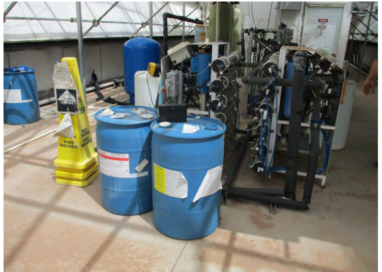
Photo 42 - View of the part of the reverse osmosis system in Greenhouse 1, along with drums of water conditioner.
