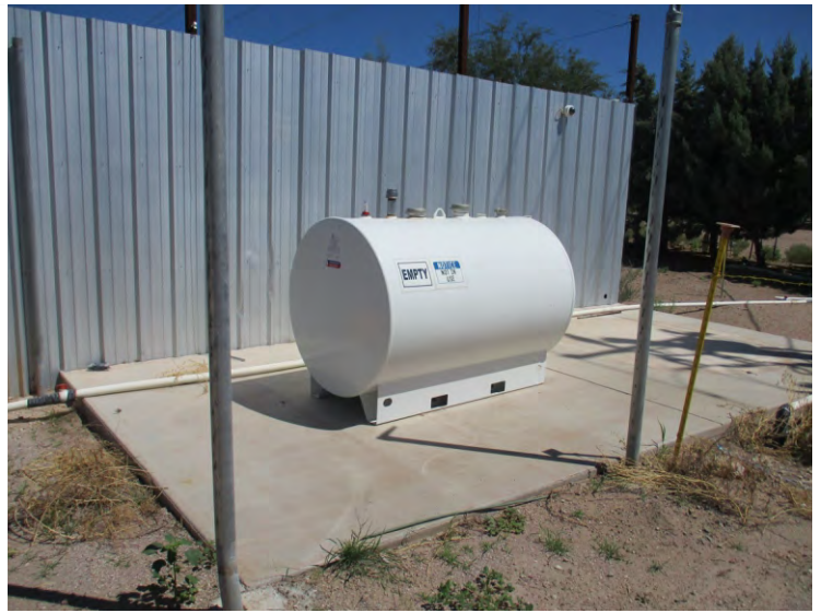
Photo 16 - View of the empty above-ground storage tank northeast of Greenhouse 2, looking northeast.
