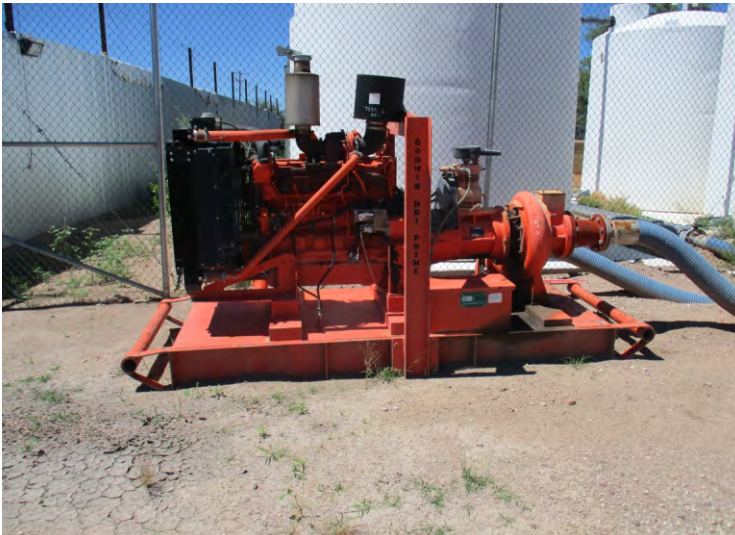
Photo 29 - View of the diesel-powered firefighting pump in the well complex.
