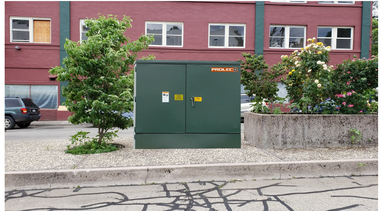
Proposed 3-phase Pad Mount Transformer
