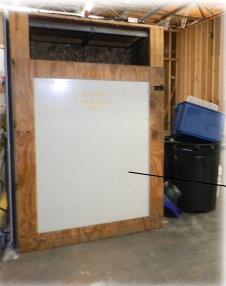
Freight Elevator is operational
