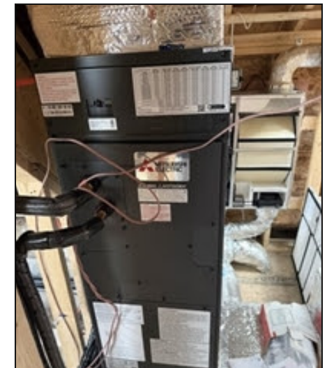
New high-efficiency HVAC
