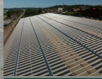
160KW SOLAR ROOFTOP
