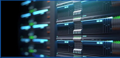
Integrated Tech and Server Room
