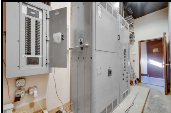
EXPANSIVE ELECTRICAL PANEL
