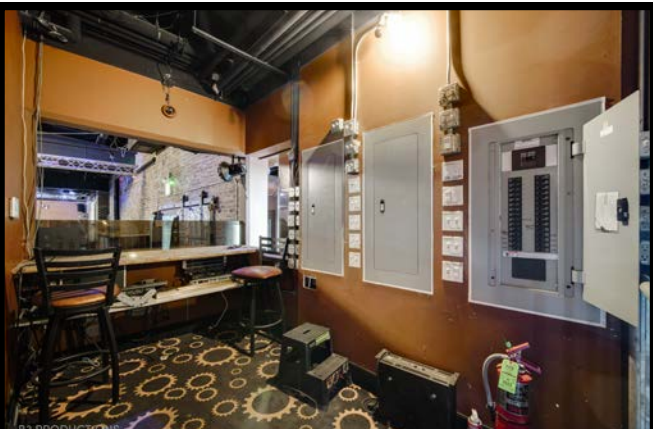
DJ BOOTH WITH ALL OF THE EQUIPMENT FACING THE LARGER ROOM
