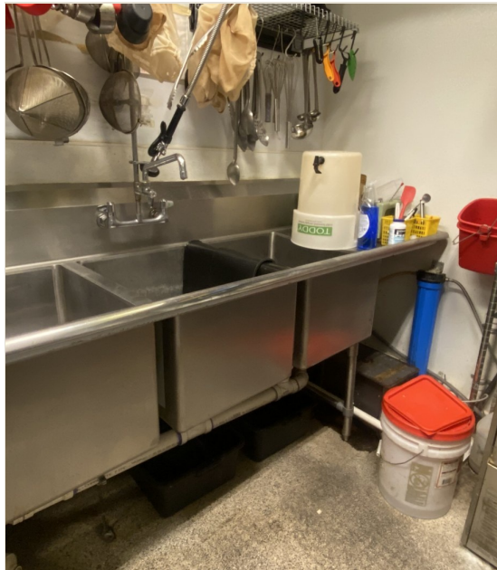
Dish Station — three-compartment sink & utensil storage
