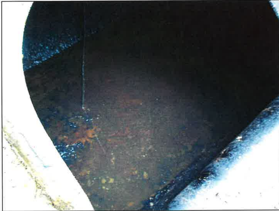
Photograph 5: View of residual material in the bottom of the tank.
