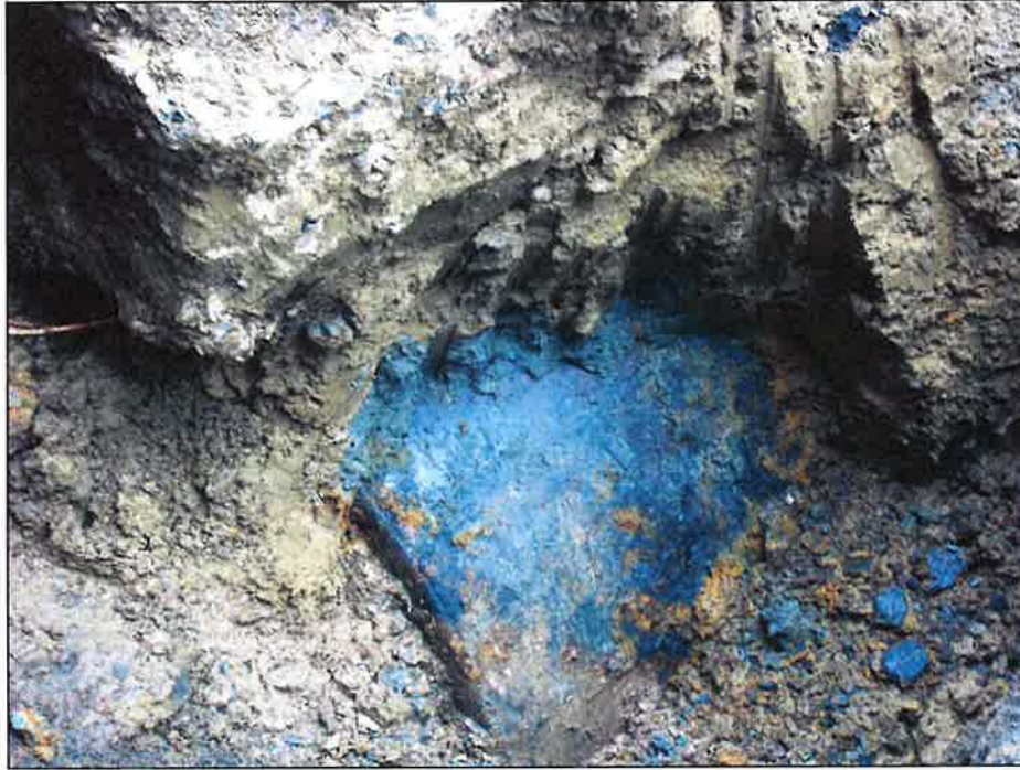
Photograph 3: View of the side of the tank after excavating alongside the concrete porch.
