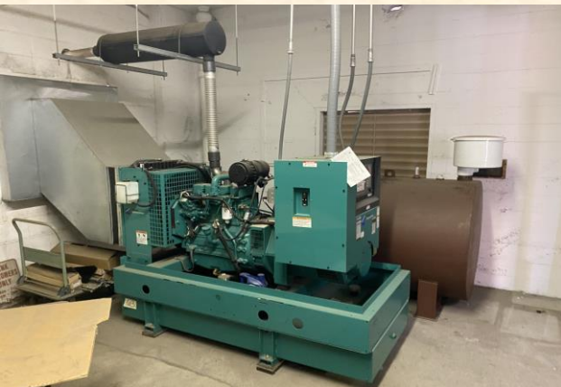
EMERGENCY POWER - BACKUP GENERATOR
