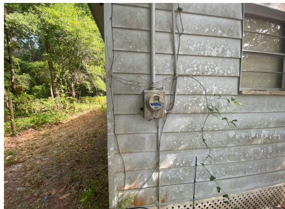
Electrical Meters SFR (Parcel Two) Photo taken June 11, 2024
