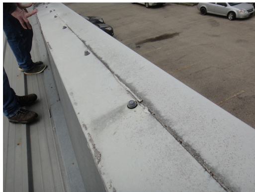
Roof coping poor
