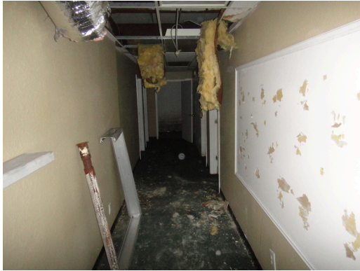
Bldg 2 interior poor
