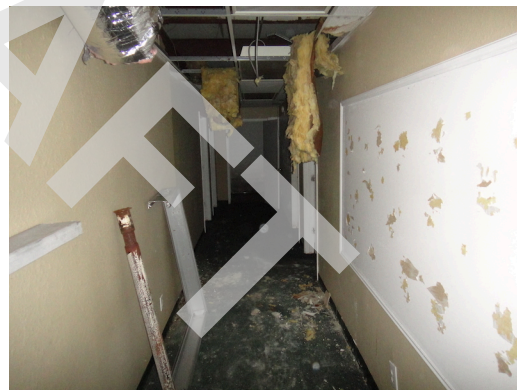
Bldg 2 interior poor
