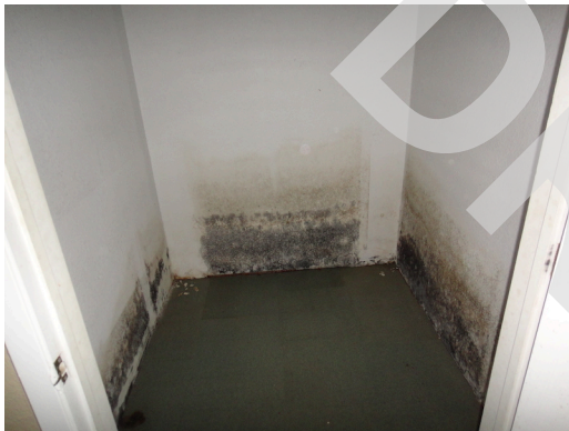
Mold damage bldg 2
