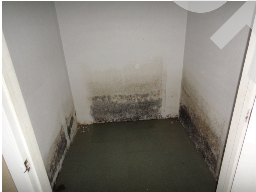
Mold damage bldg 2
