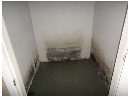
Mold damage bldg 2
