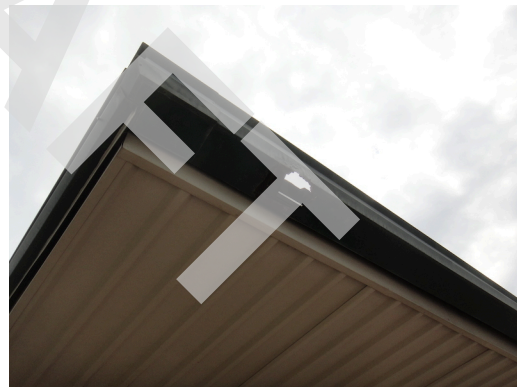
Damaged gutter areas
