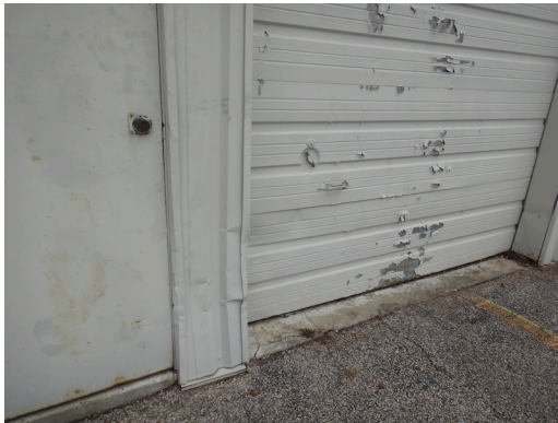
Fair to poor finishes
