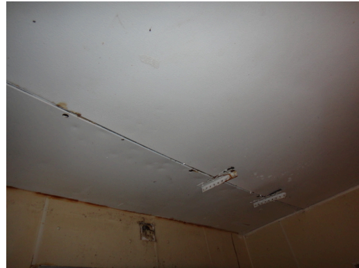
Roof leak bldg 1
