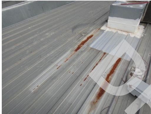
Roof surface rust bldg 1
