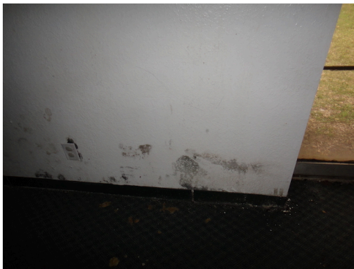
Moisture damage bldg 2
