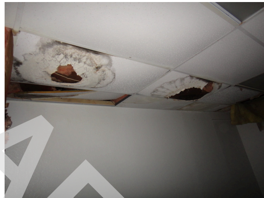
Past roof leaks bldg2
