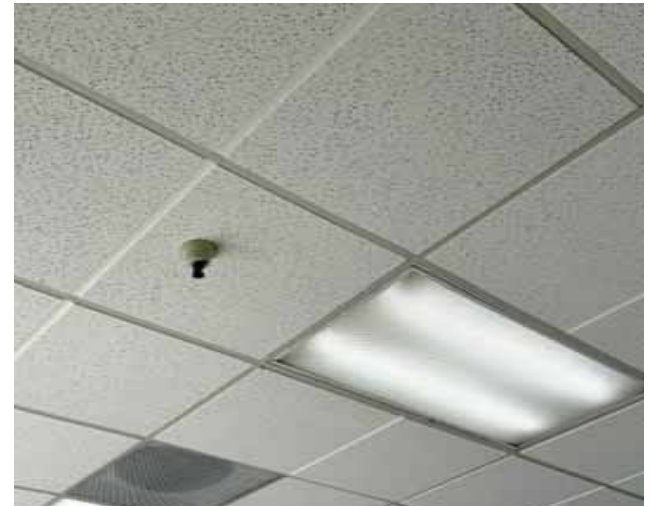
3093 McKee Road - Fire Sprinklered
