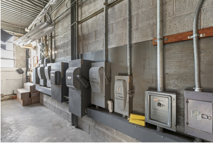
Heavy Power—400 Amp, 3 Phase
