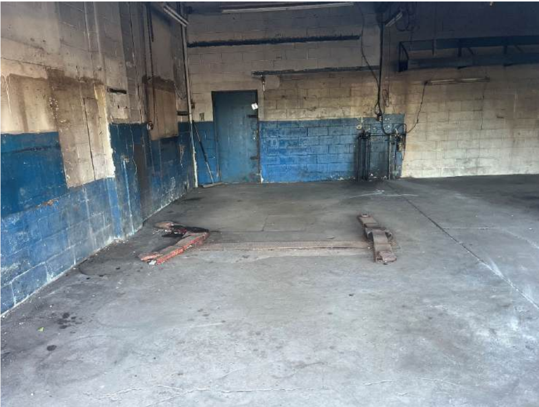
Photo 10 – In-ground hydraulic lift
