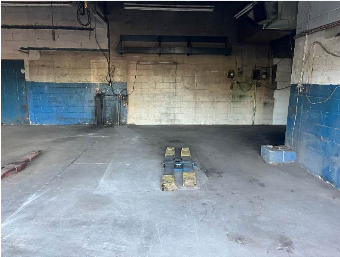
Photo 9 – In-ground hydraulic lift
