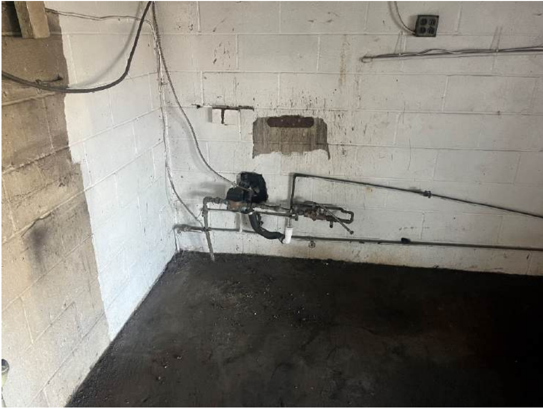
Photo 11 – Building water meter
