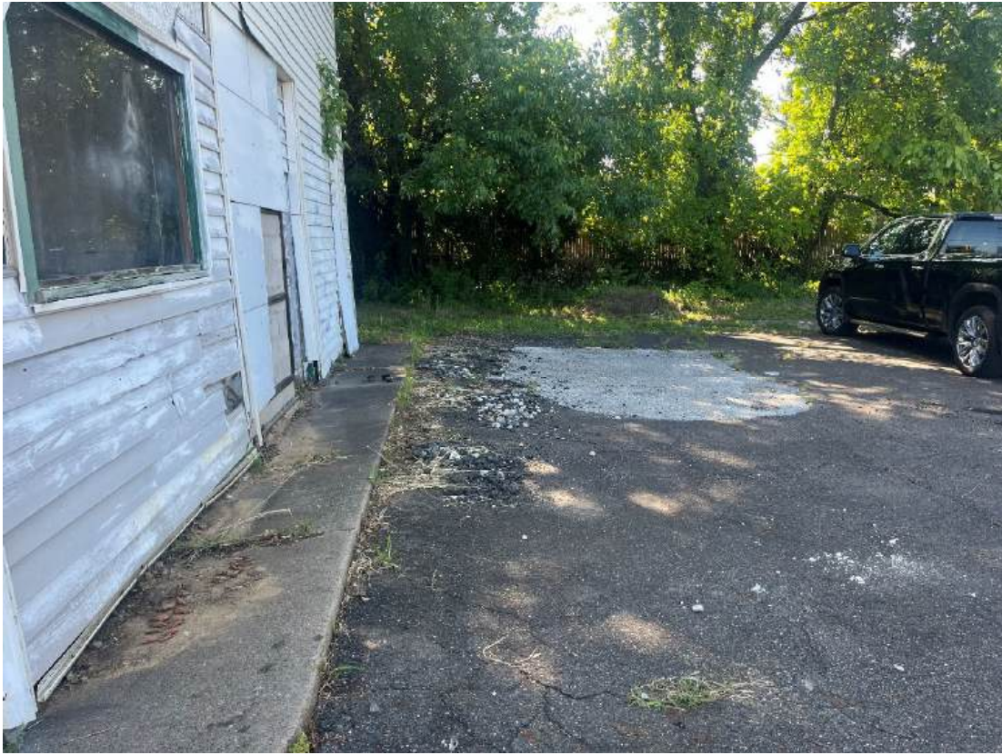
Photo 7 – Disturbed blacktop to the south of the building
