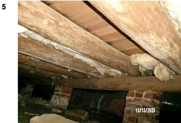
decayed round floor joist, note mold on joist under chapel
