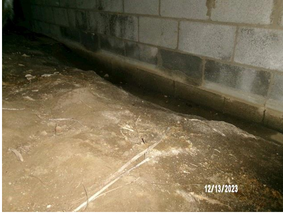
CRAWL SPACE: missing vapor barrier, damp foundation walls.
