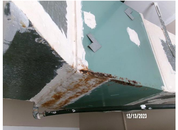
COOLING - HEAT PUMPS: rust/deteriorated evaporator coil cabinet
