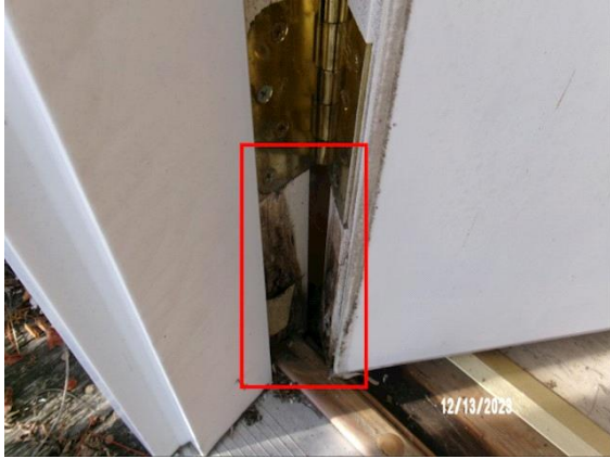
DOORS - EAST WING: decay in kitchen door & jamb
