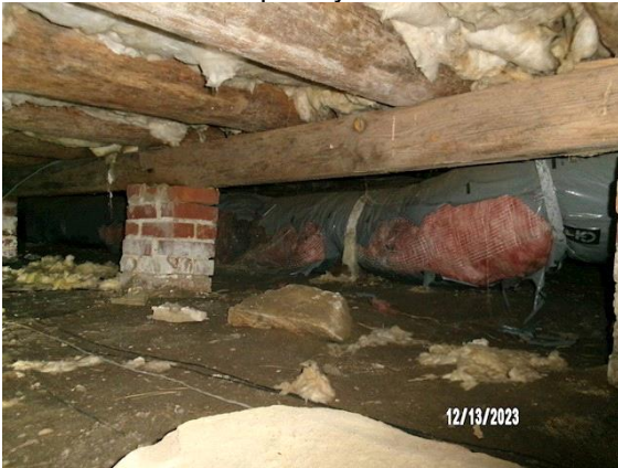
HVAC DISTRIBUTION: Typical torn duct vapor barrier, hole torn in duct, duct on ground
