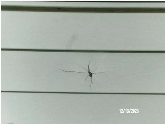
EXTERIOR SURFACE: hole in siding
