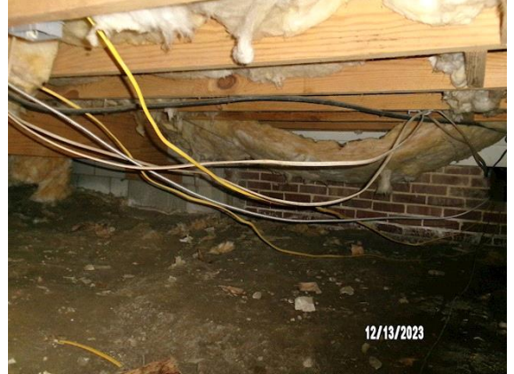
typical wires dangling thru crawl spaces
