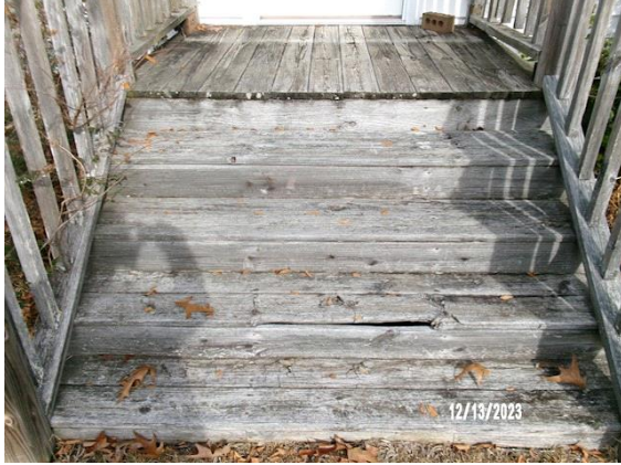
FLATWORK / SIDEWALKS: general decay / deterioration at back wood steps
