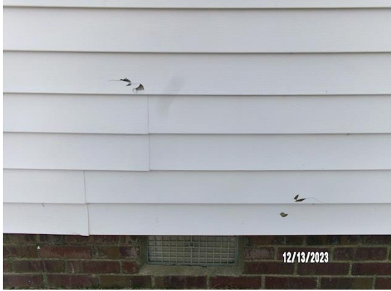
EXTERIOR SURFACE: holes in siding
