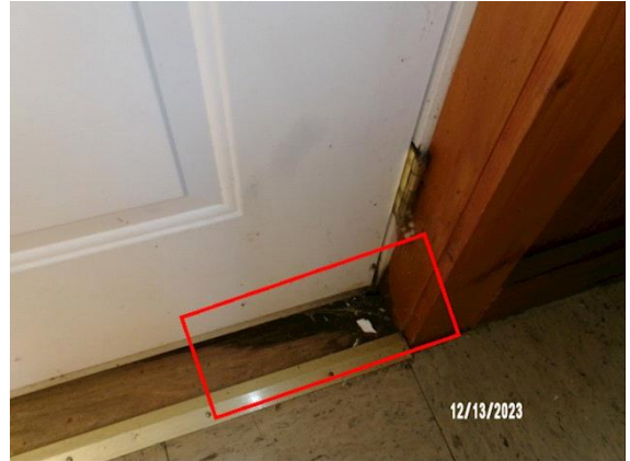
DOORS - EAST WING: water intrusion along kitchen door
