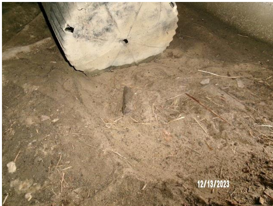
CRAWL SPACE: missing vapor barrier, wet crawl space earthen floor
