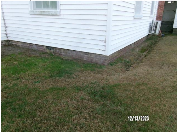
GRADING / DRAINAGE: typical negative grade along foundation
