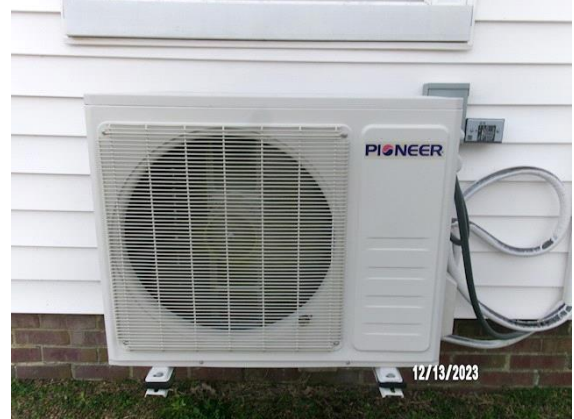
HVAC 1: typical mini system heat pump
