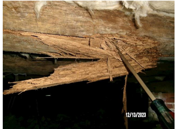
STRUCTURAL FRAME AND BUILDING ENVELOPE: probing a typical round timber floor joist
