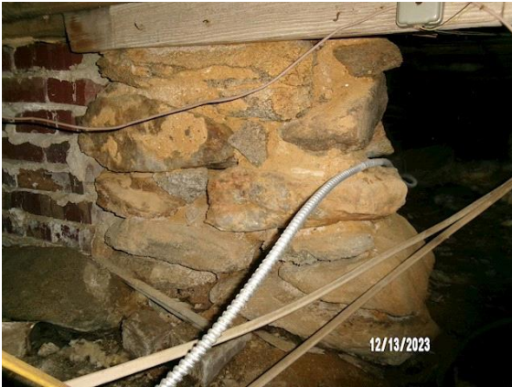
STRUCTURAL FRAME AND BUILDING ENVELOPE: typical stone pier with deteriorated mortar
