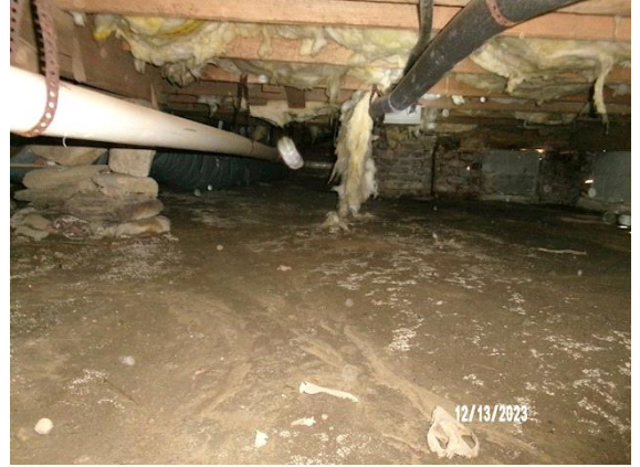
CRAWL SPACE: erosion in wet crawl space earthen floor, also missing vapor barrier
