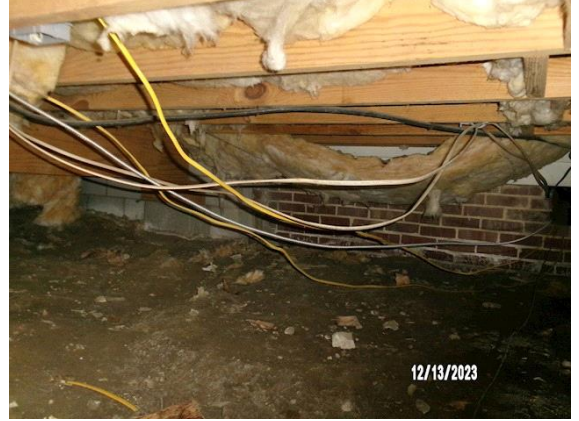
CRAWL SPACE: fallen insulation, damp earthen floor
