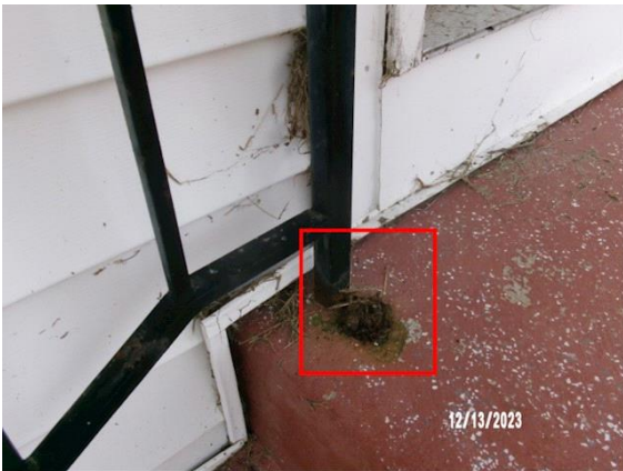
FLATWORK / SIDEWALKS: left handrail post at front entry rusted thru
