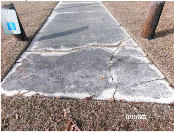
FLATWORK / SIDEWALKS: typical cracked/broken concrete w/vertical offset
