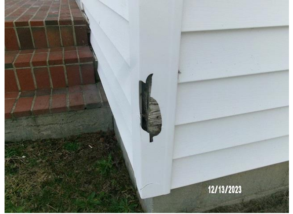
EXTERIOR SURFACE: hole in siding corner post
