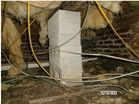
CRAWL SPACE: typical fallen floor insulation
