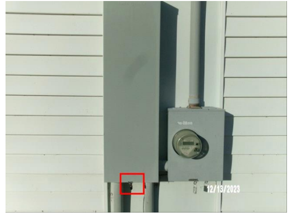
Electrical: main electrical panel - pad locked
