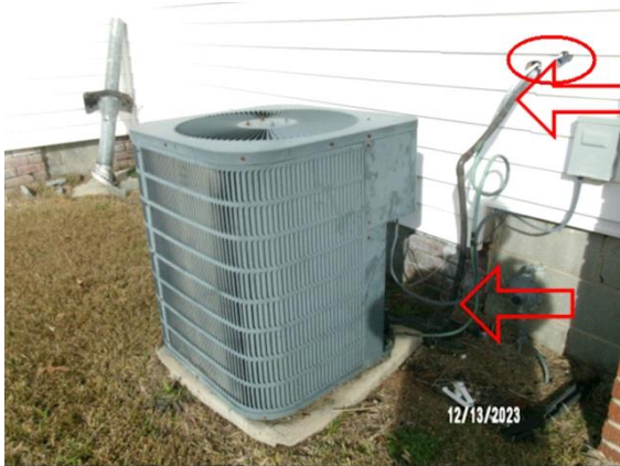
COOLING - HEAT PUMPS: exposed suction line, missing sealant at siding
