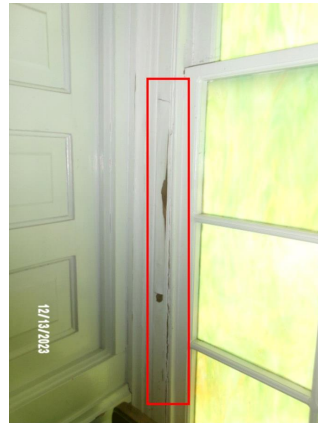
CHAPEL: WDI damage left facing window
