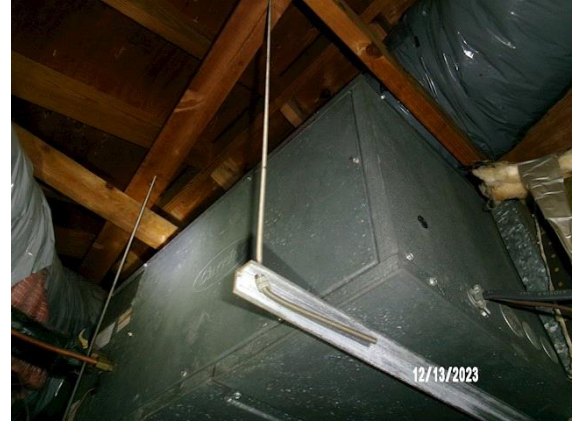
Cooling - Goodman: air handler located above west wing class room ceiling
