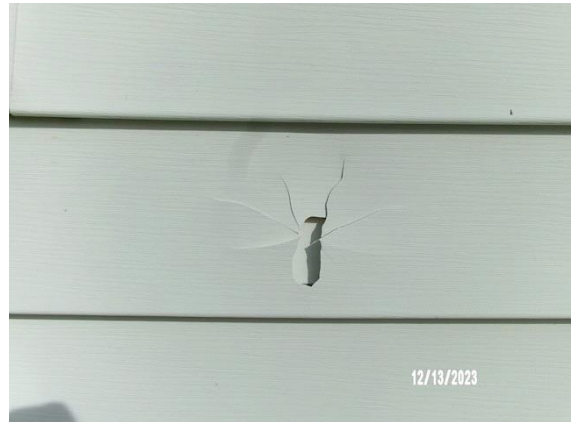
EXTERIOR SURFACE: hole in siding
