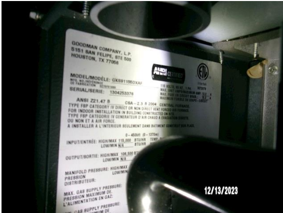
HVAC 2: Goodman furnace data plate
