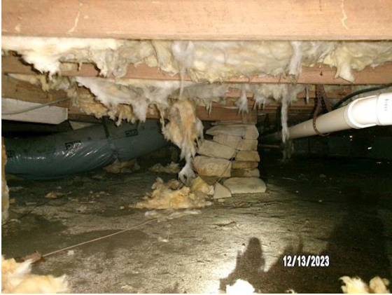
CRAWL SPACE: fallen , stringy insulation (moisture caused) missing vapor barrier
