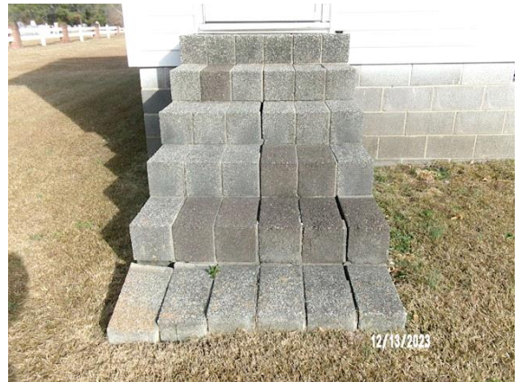
FLATWORK / SIDEWALKS: separation / settlement at back right steps, no handrail
