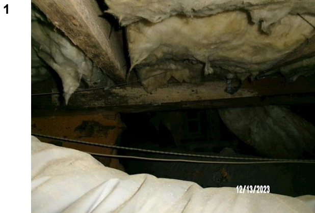
mold covered floor framing - crawl space
