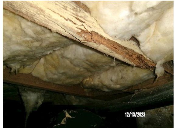
STRUCTURAL FRAME AND BUILDING ENVELOPE: probing a mold covered floor joist
