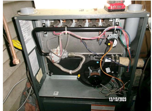
HVAC 2: Goodman furnace
