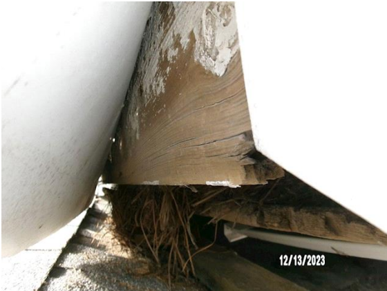
EXTERIOR SURFACE: loose aluminum trim at water table
