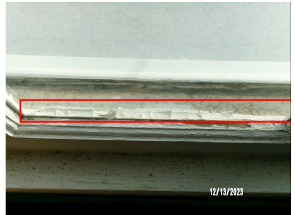
FENESTRATION SYSTEMS: brittle / cracked glazing putty
