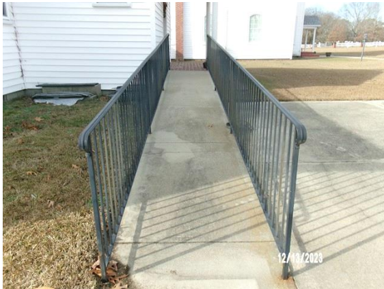
FLATWORK / SIDEWALKS: loose handicap railings
