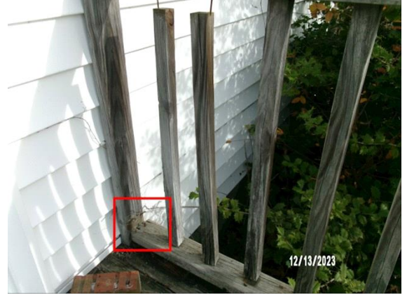
FLATWORK / SIDEWALKS: failed nail connection at back wood steps handrail
