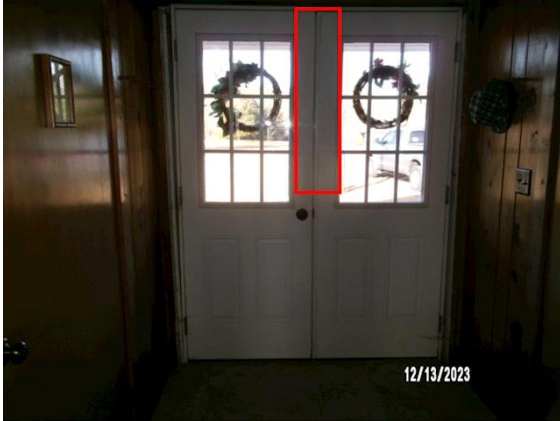
Doors - East Wing: doors do not seal along astragal
