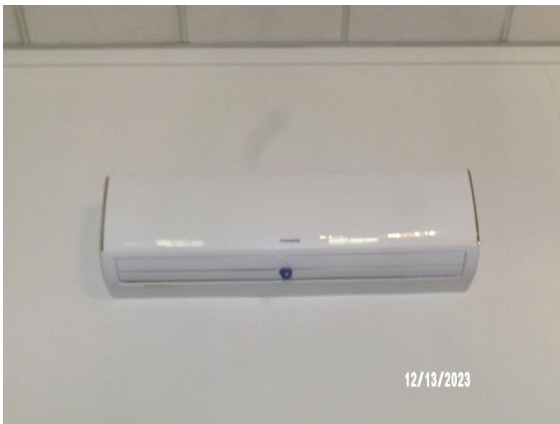
HVAC 1: typical mini system air handler
