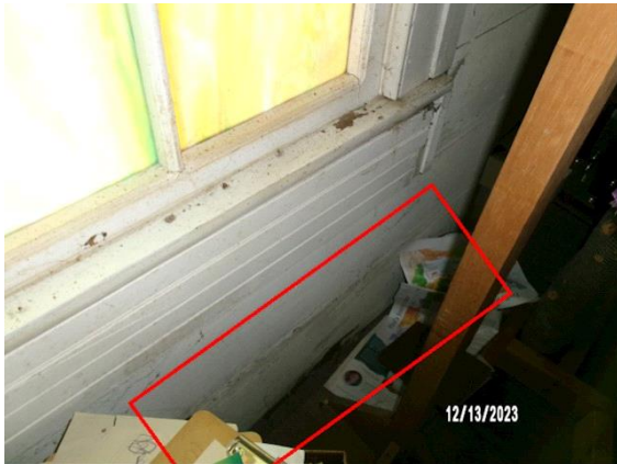
CHAPEL: WDI damage under front window
