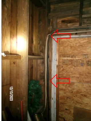
WDI activity in furnace closet
