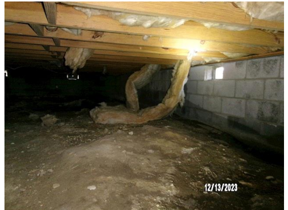
CRAWL SPACE: typical fallen floor insulation, missing vapor barrier
