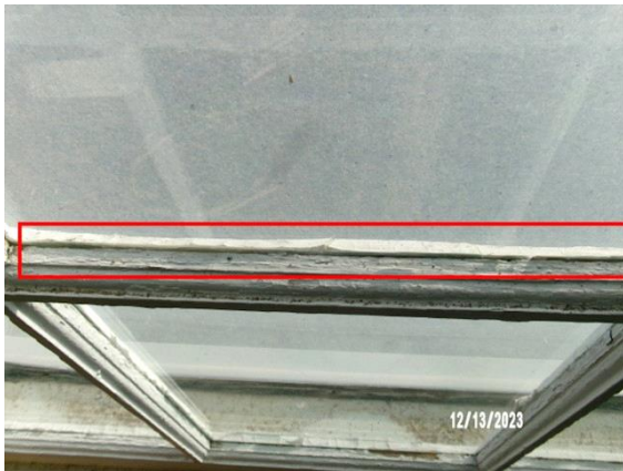
FENESTRATION SYSTEMS: brittle / cracked glazing putty
