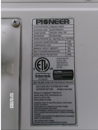
HVAC 1: typical mini heat pump data plate
