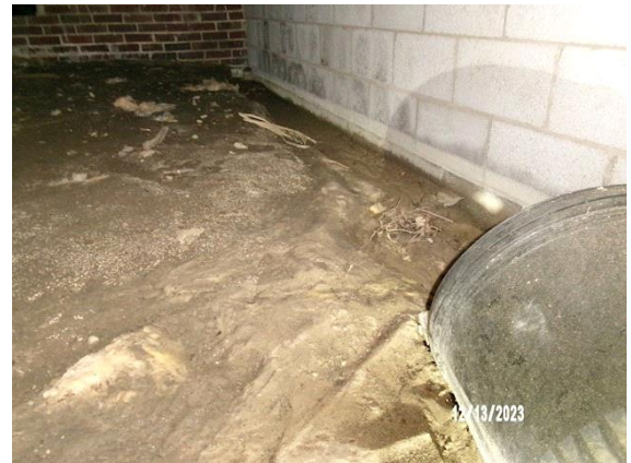
CRAWL SPACE: erosion in wet crawl space earthen floor, also missing vapor barrier
