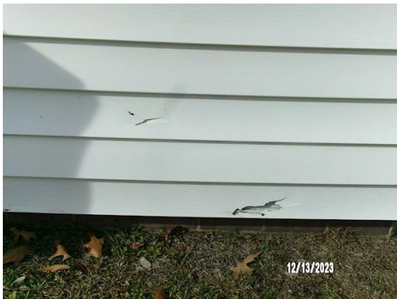
EXTERIOR SURFACE: holes in siding
