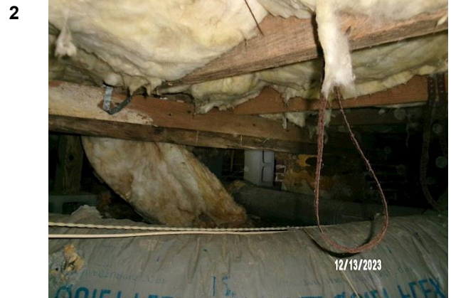
mold covered floor framing - crawl space
