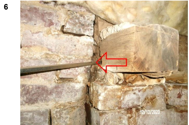
probe pushed through outer floor support - crawl space
