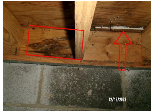
DOORS - WEST WING: decayed sub floor & band joist under door
