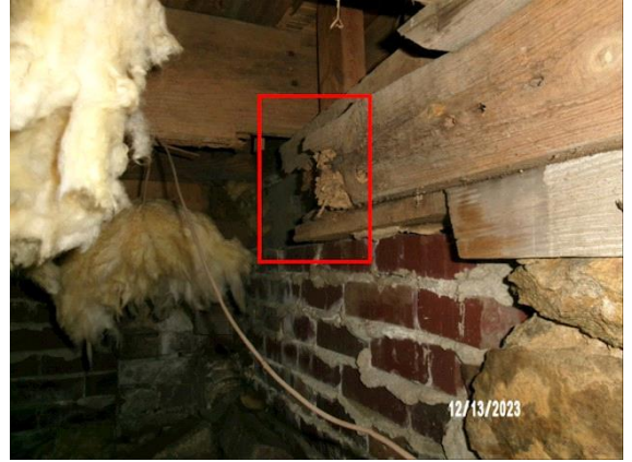
STRUCTURAL FRAME AND BUILDING ENVELOPE: decayed/WDI damage joist
