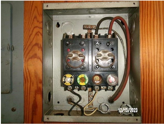
Electrical: fused sub panel
