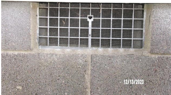
EXTERIOR FOUNDATION: typical vent missing a vent door/handle
