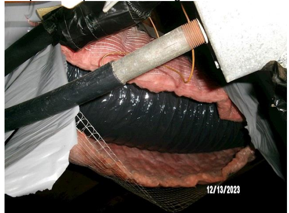
HVAC DISTRIBUTION: typical torn vapor barrier, missing duct insulation
