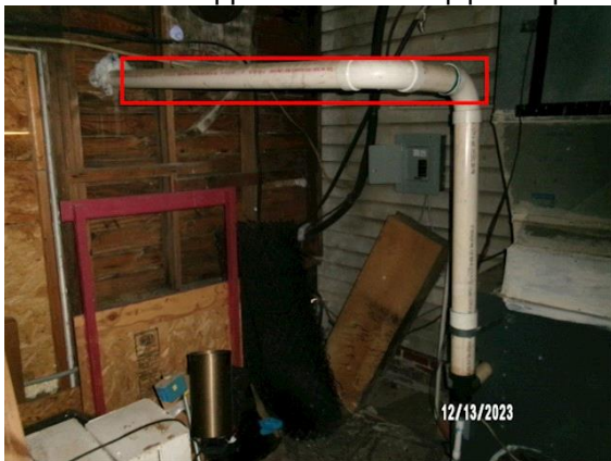
DRAFT CONTROL / VENT GOODMAN FURNACE: no support strapping
