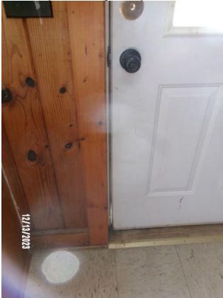
DOORS - EAST WING: kitchen door does not seal
