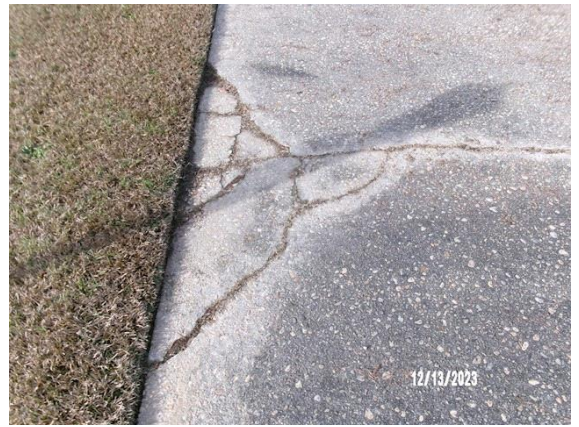
FLATWORK / SIDEWALKS: typical cracked/broken concrete
