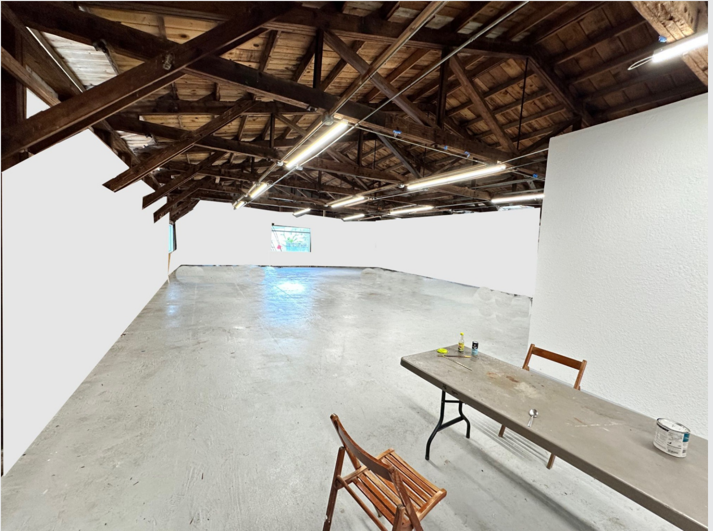
Main space: 2534 sf incl. office This picture is photoshopped, the wall will be drywalled shortly
