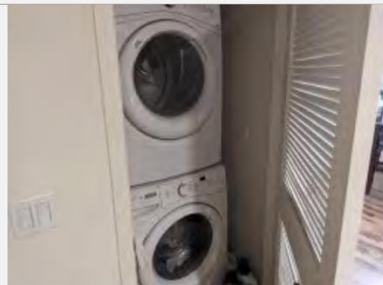
IN UNIT LAUNDRY (BLD A/UNIT 110)
