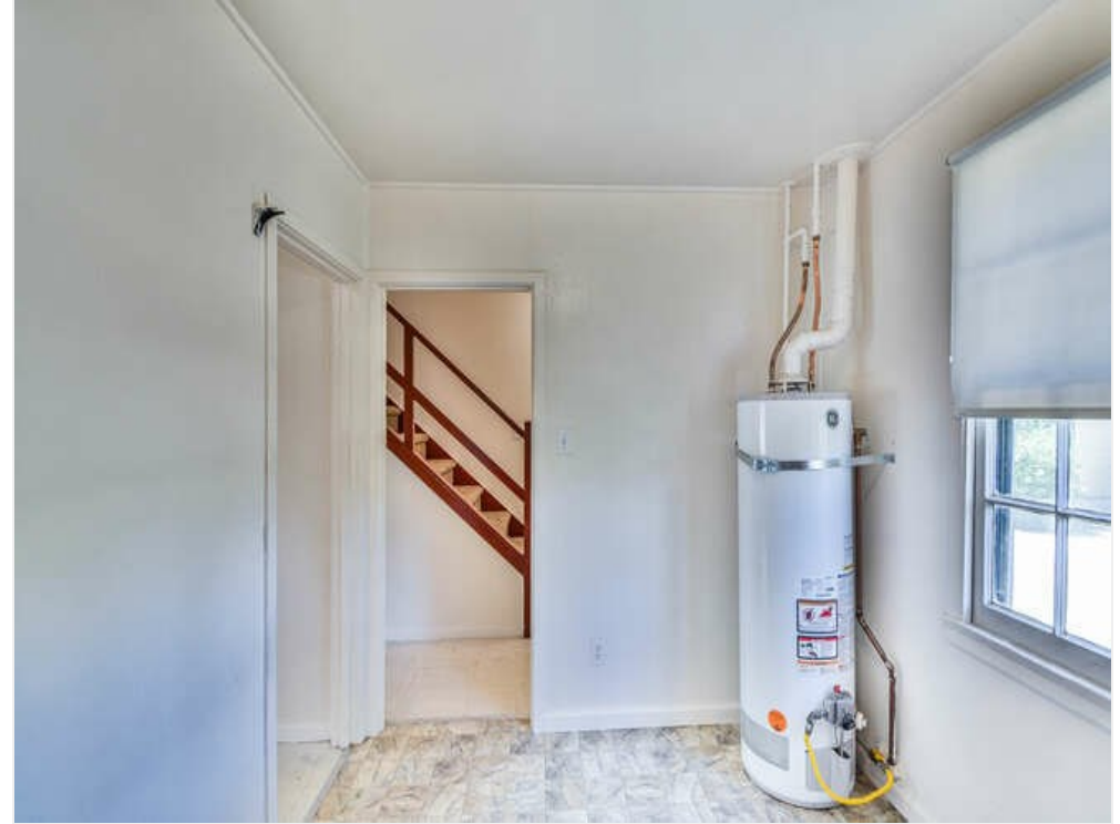
1572 and 16081614 E 6th St-small-038-046-Water Heater-666x445-72dpi
