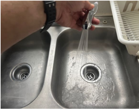
General Info: Under Sink Pictures Kitchen
