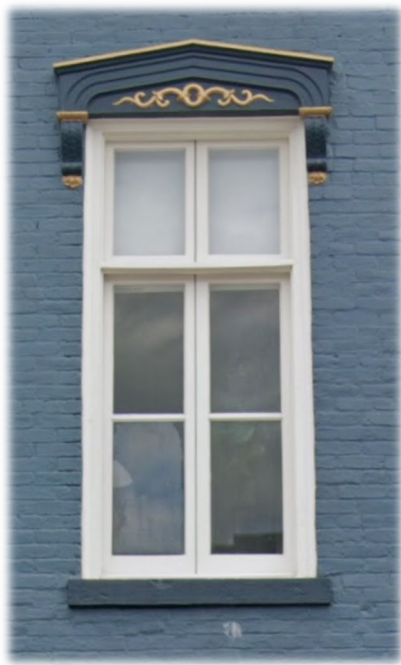
An example of a restored window at the Coleman-Allen building at 1-11 E. Main Street
